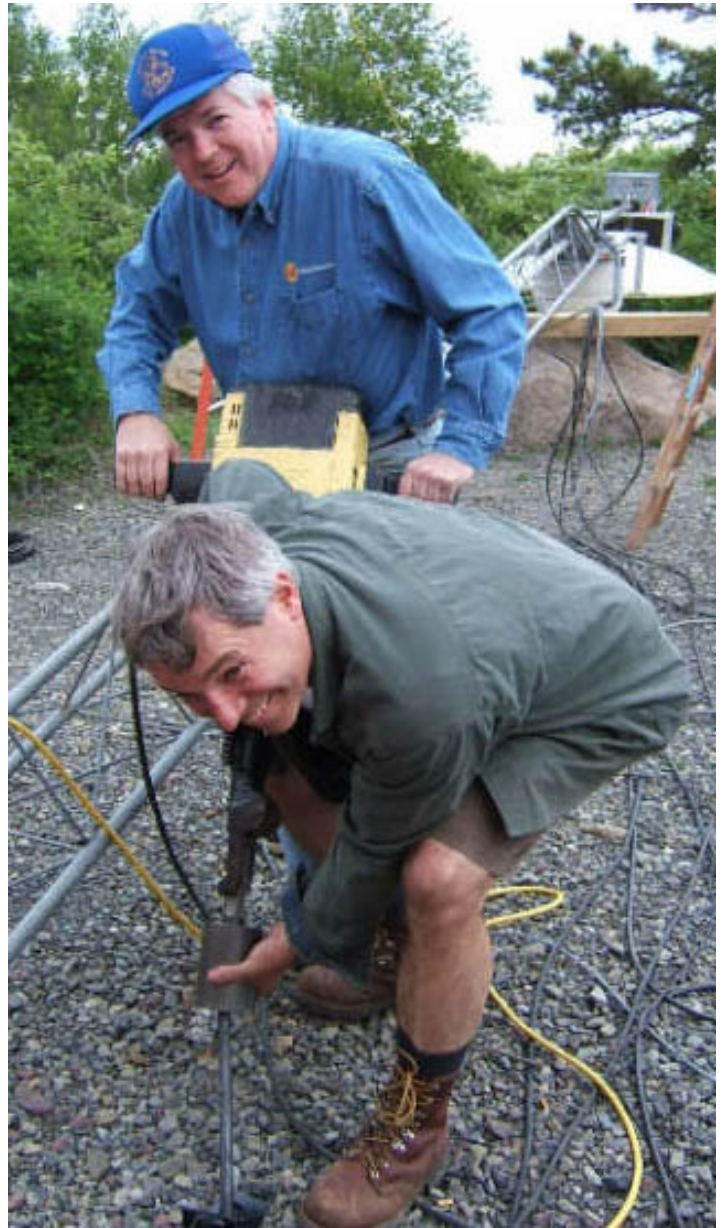
Having the right tools for the job certainly helped us make sure the towers stayed up with all the wind. Here are WA3NUF and KB3XG using the electric jackhammer to set anchor stakes for one of the microwave towers.
